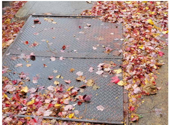
A possible coal delivery chute noted at a business along Davis Avenue
