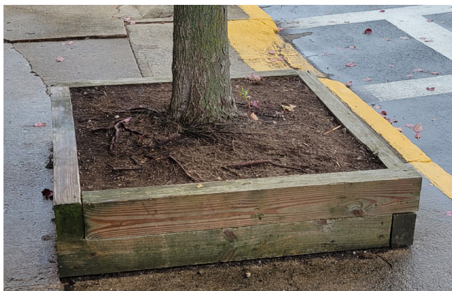
A large maple tree boxed in with a timber structure exhibits signs of restricted growth on 3rd Street.
