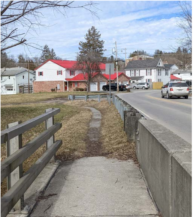
Existing vehicular bridge at Industrial Park Road provides a safe pedestrian crossing.
