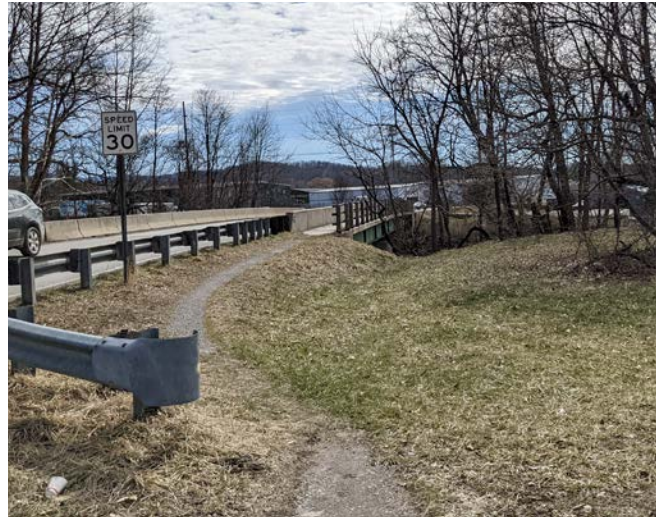
A desired path has developed on either side of the Industrial Park Rd. bridge highlighting the need for better connections to these areas.
